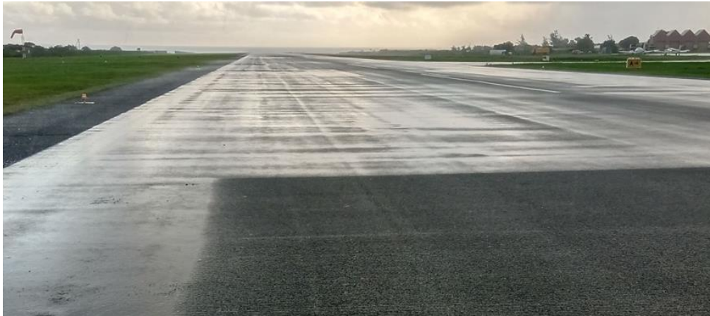
Grooving being implemented on a newly paved runway shows the impact on runway surface condition.
